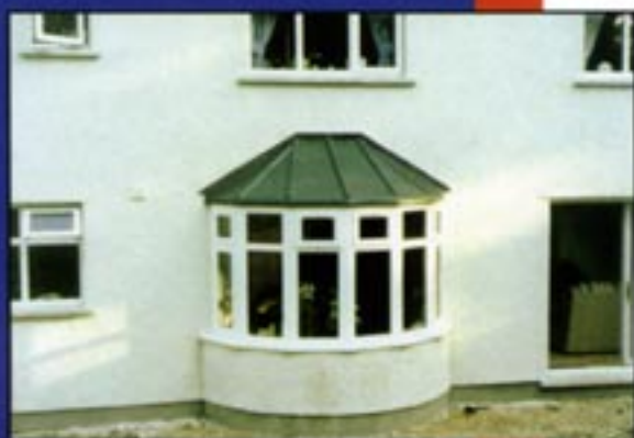
Above: An example of pre-fabricated lead-effect cladding on a steeply pitched roof section.
